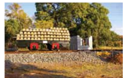
Railway line: Load tests on the section of railway line constructed for research purposes on the University of Pretoria's Research Farm.
