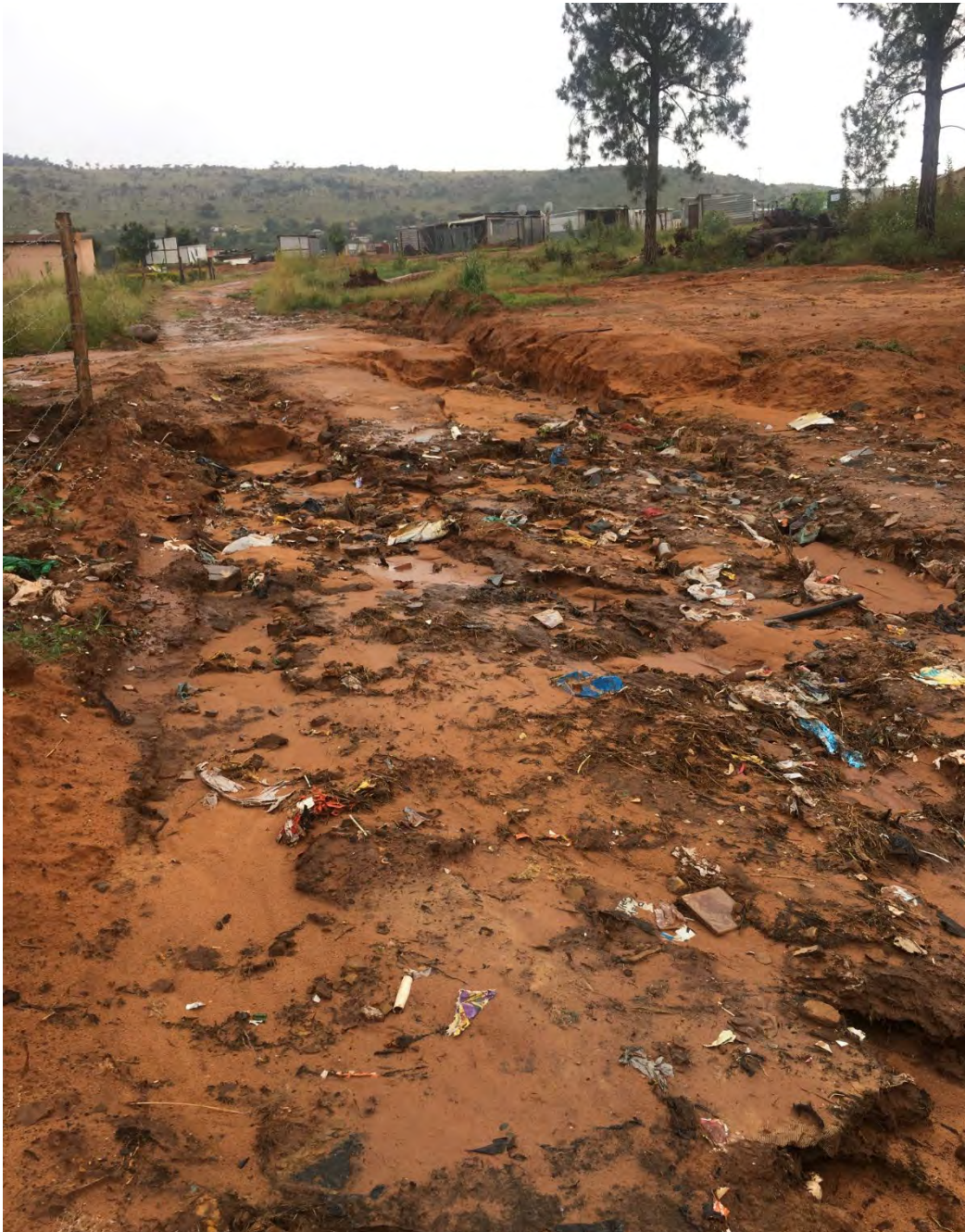
Image above: A section of the road to Dikeledi's house has been washed away
